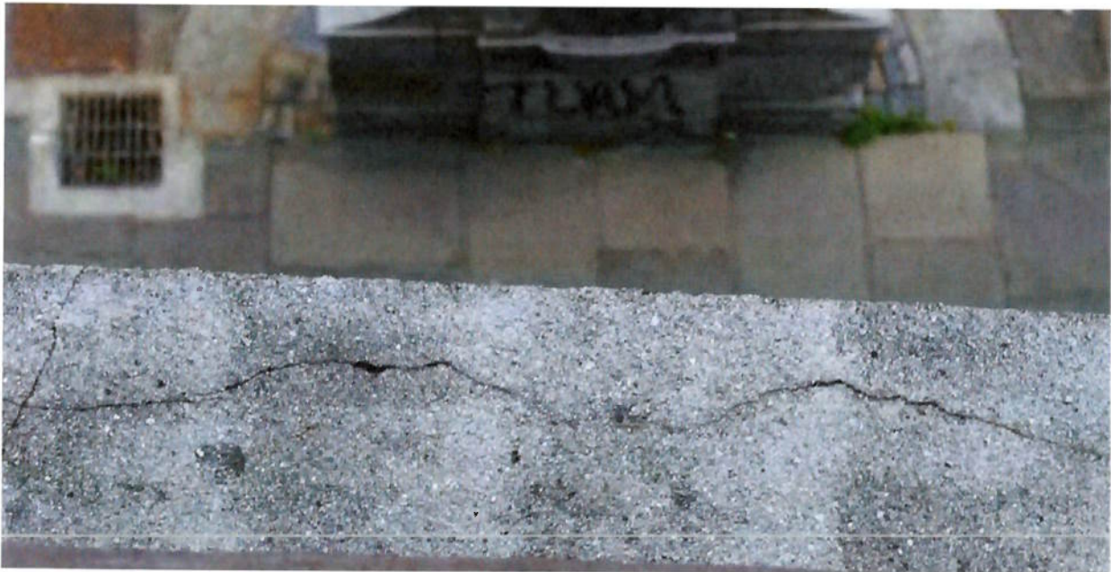
Figure 27. Cracks through the rendered cornice (viewed from the roof).
