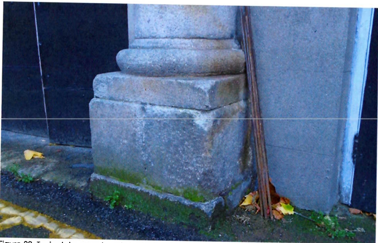
Figure 39. Typical damage to column bases
