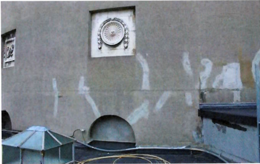
Figure 8. Defective cement-based render at roof level. Area to be re-rendered.
