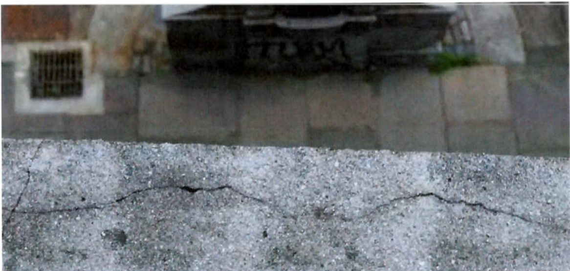
Figure 24. Cracks through the rendered cornice (viewed from the roof).
