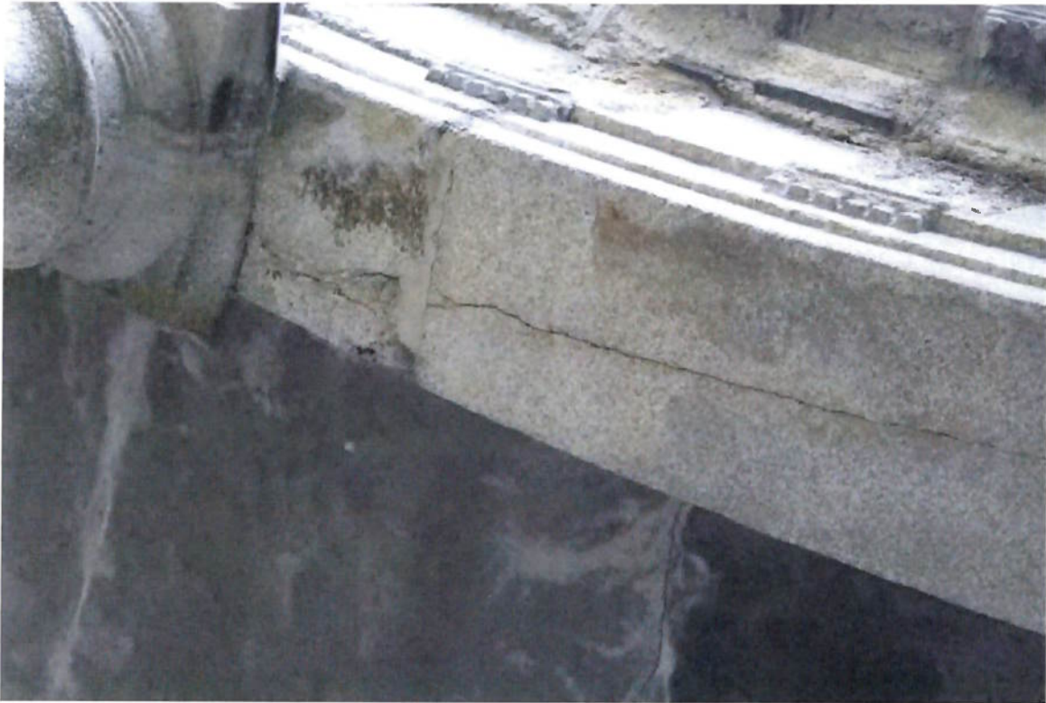
Figure 17 Cracks to the granite soffit. All soffit granite to be inspected by a conservation accredited engineer.
