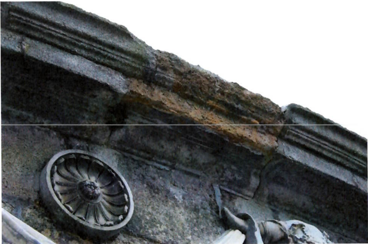
Figure 8. Deteriorated section of granite cornice.
