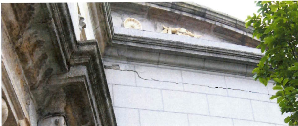
Figure 25. Horizontal cracking and detaching render to the East façade.
