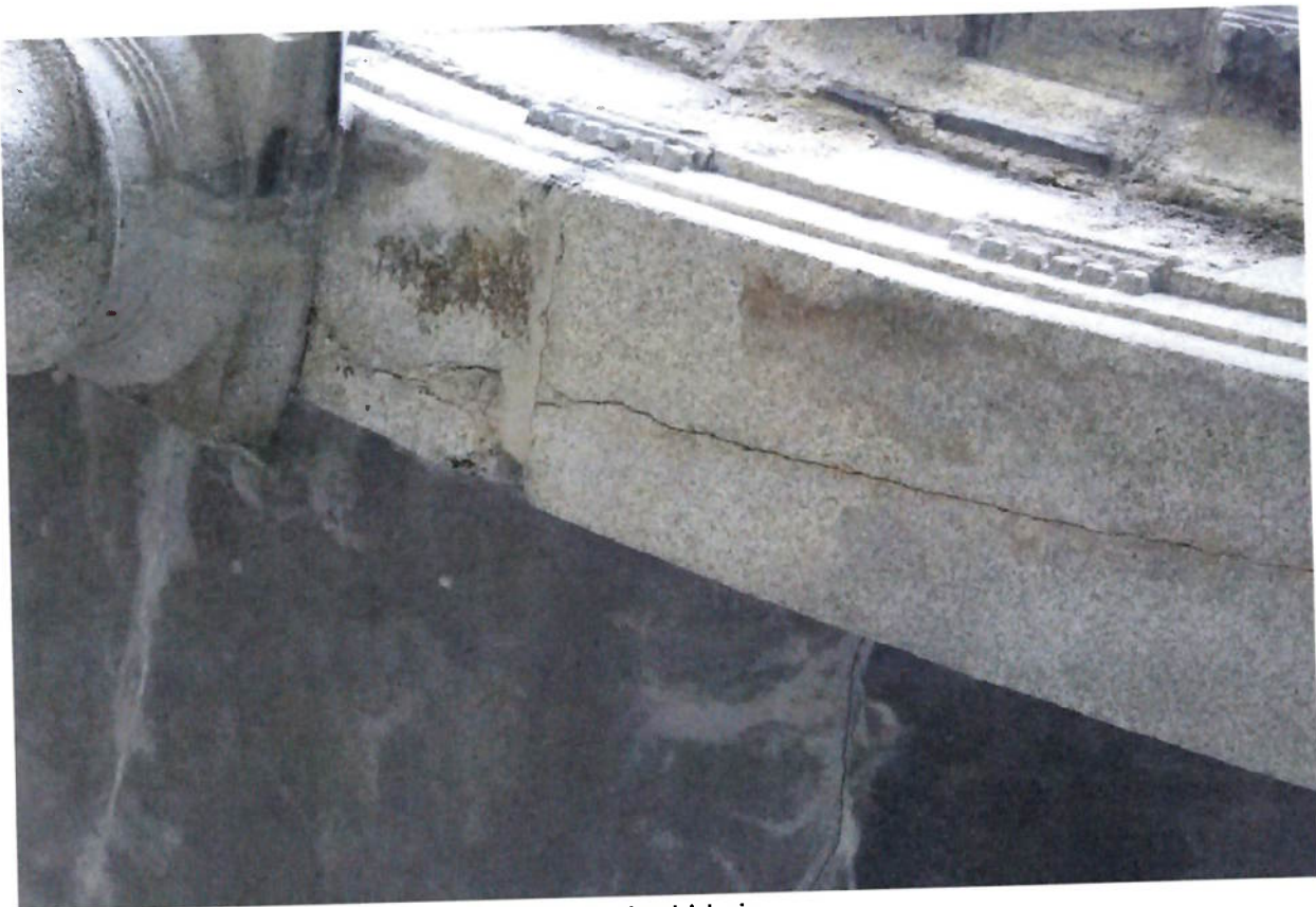
Figure 20. Cracks to the granite soffit that may be historic.
