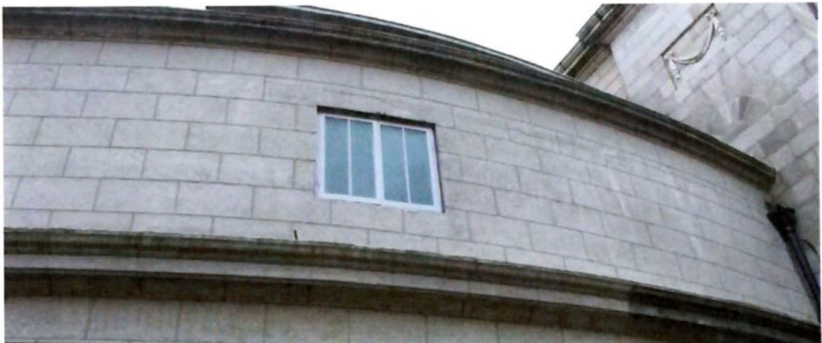
Figure 23. Continuation of the horizontal cracking to the East Elevation
