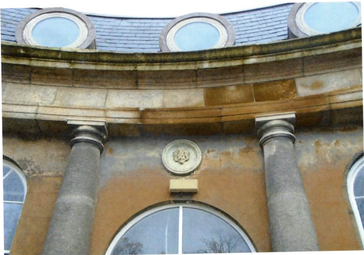
Figure 36. Further evidence of staining
