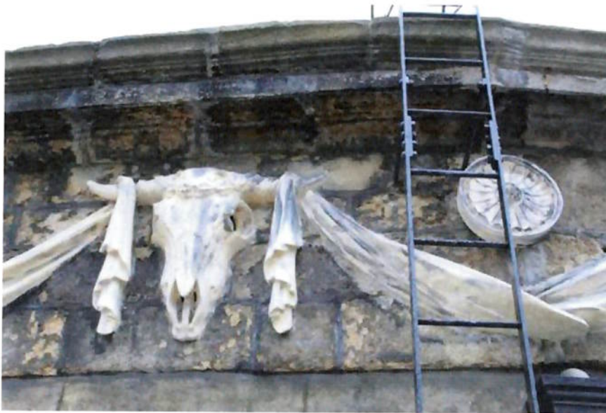
Figure 3. Replaced 'new' Coade Stone elements from a previous repair scheme. The moulds are still available for the replacement Coade Stone elements required.
