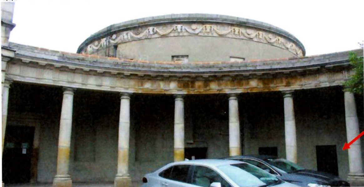
Figure 15 Arcade link to the Rotunda Hospital with the Rotunda Theatre building behind. Left had side was subject to a cleaning trial by Thomann-Harry. This has proved to be too severe and we do not recommend using it.
