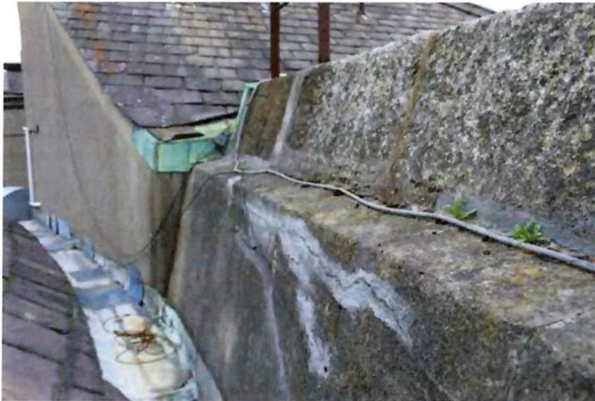
Figure 6. Inner parapet of the rotunda theatre building cracked cement render. Very deteriorated sections area to be repaired.
