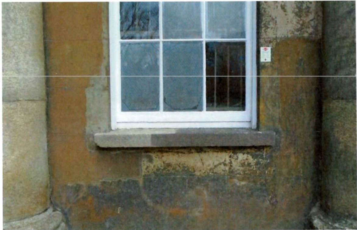
Figure 28. Current condition of rendered façade between engaged columns. Part of the sill has been cleaned using the Façade Gommage System, which is inappropriate.
