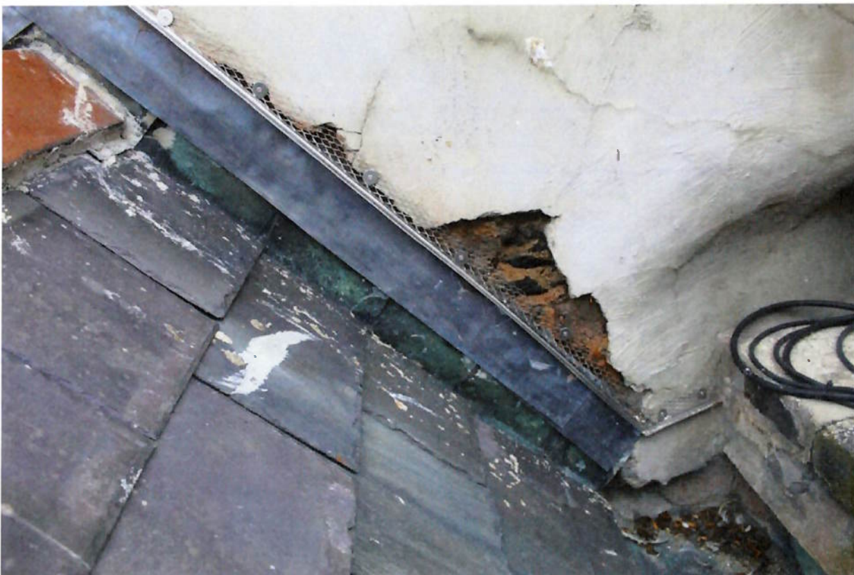
Figure 17. Defective render and flashing allowing water ingress.
