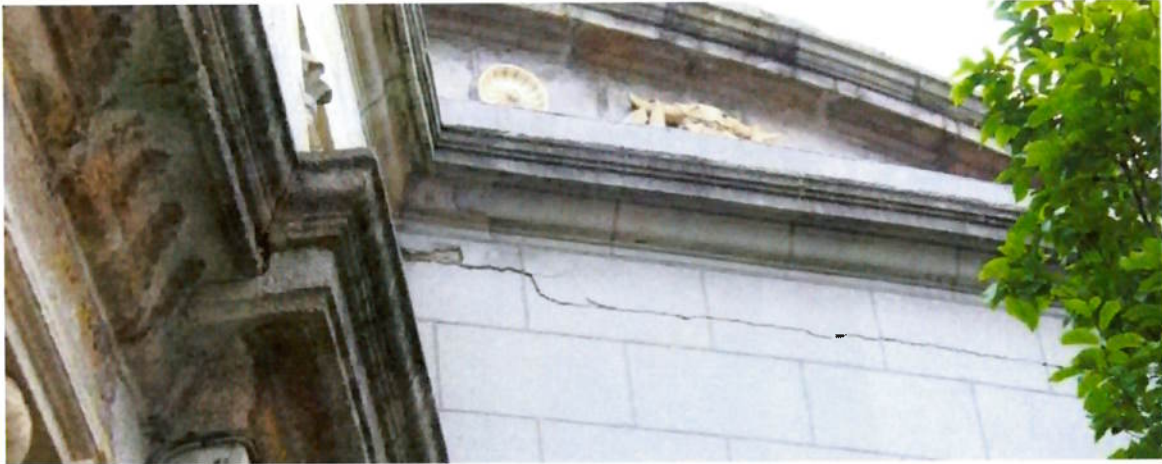
Figure 22. Horizontal cracking and detaching render to the East façade. Investigate cause under the supervision of a conservation accredited structural engineer.
