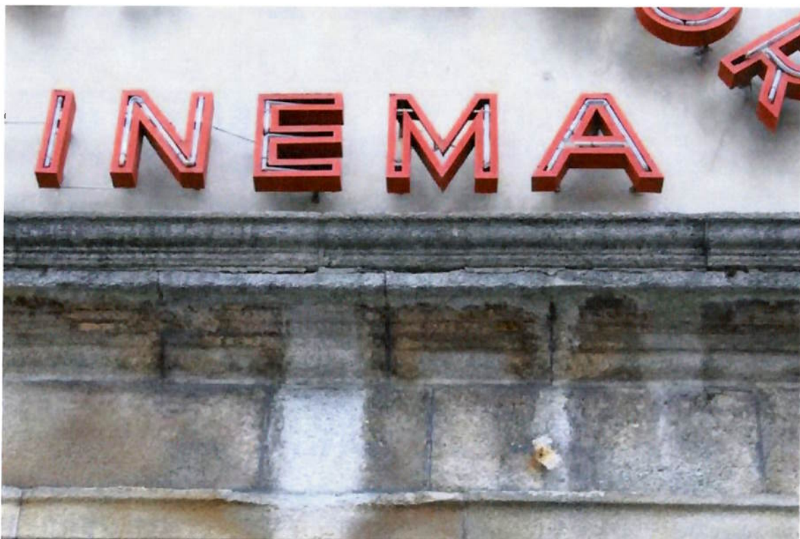
Figure 21 Poor condition of the underside of the granite cornice. Section of soffit granite to be replaced and all joints to be repointed with lime mortar.
