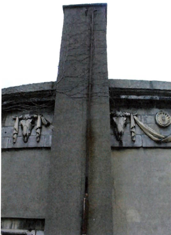
Figure 10. Defective render to chimney.
