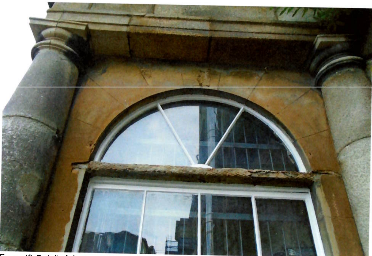
Figure 43. Detail of damaged timber lintel
