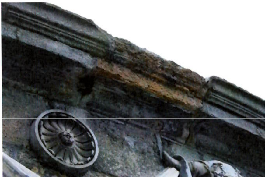
Figure 5. Deteriorated section of granite cornice to be replaced in Ballyknockan (Wicklow) Granite to match original.
