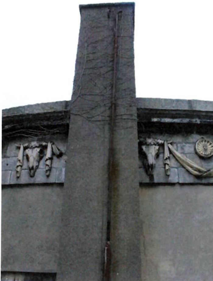
Figure 7. Defective render to chimney. Pipe to be removed and chimney re-rendered.
