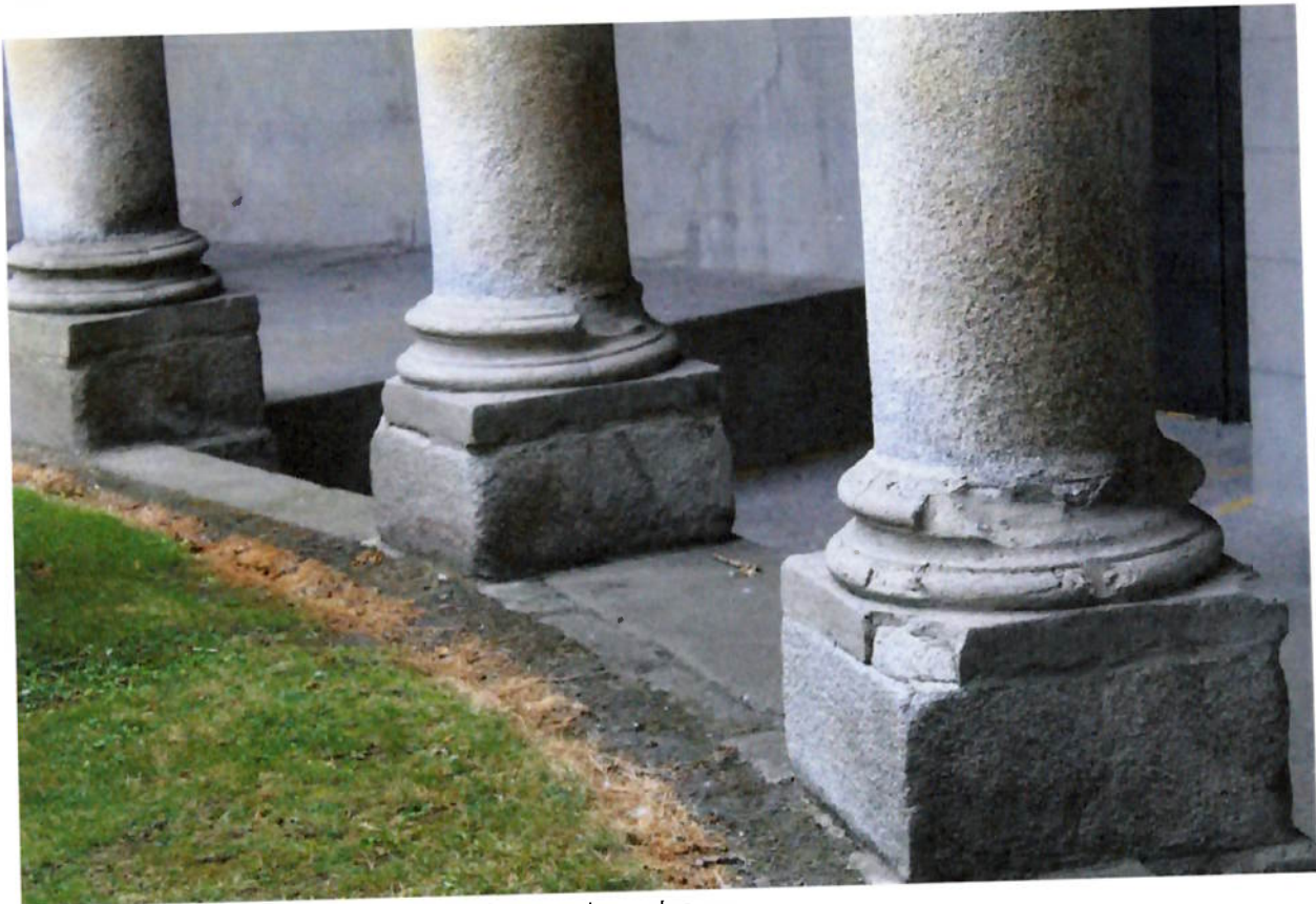
Figure 21. Deteriorating render repairs to column bases.
