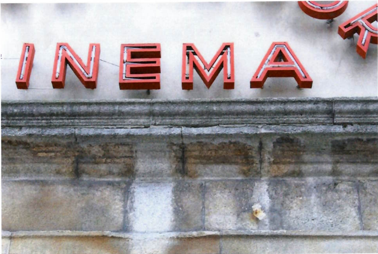
Figure 24. Poor condition of the underside of the granite cornice.
