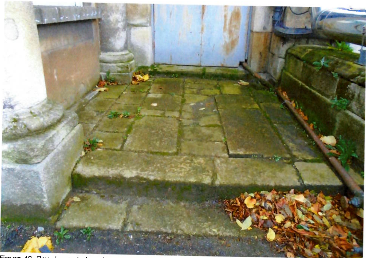
Figure 42. Flagstones to be cleaned and repointed
