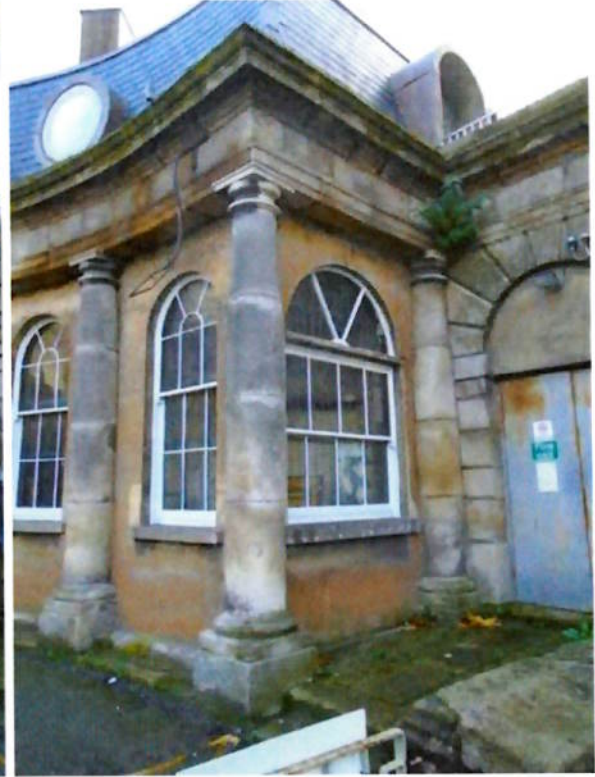
Figure 27. Altered window has an exposed timber head
