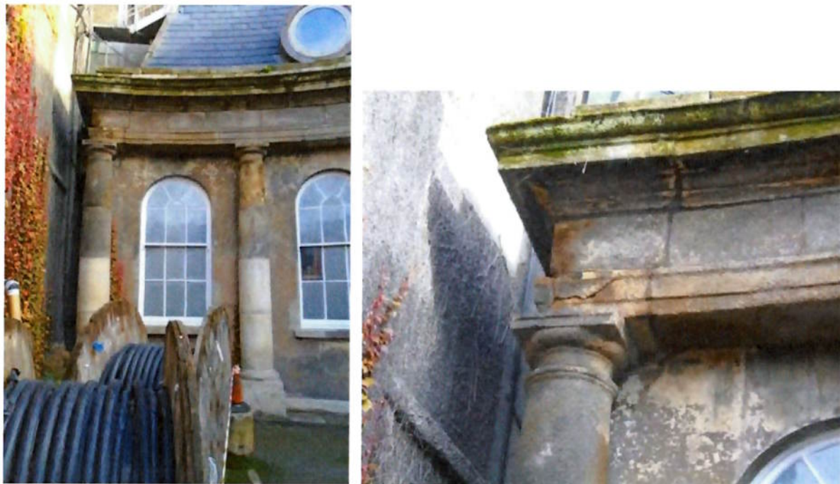
Figure 25 a & b. First bay of the façade has some cleaning samples to the lower sections of the columns, carried out previously, again using the Façade Gommage system, which is inappropriate and too aggressive. The granite at the top left hand side is damaged and requires a stone indent.
