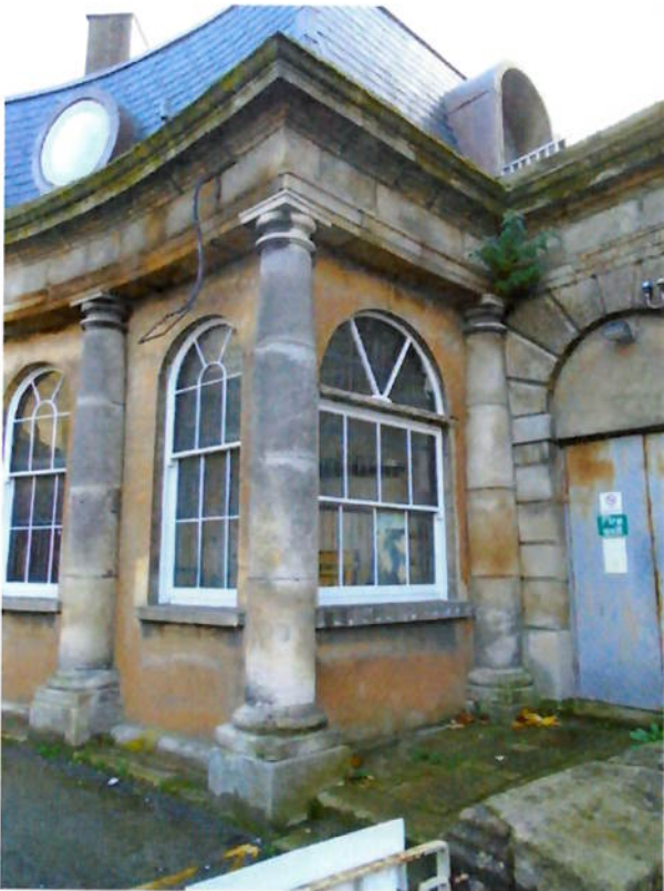
Figure 30. Corner showing inserted window with exposed damaged timber lintel
