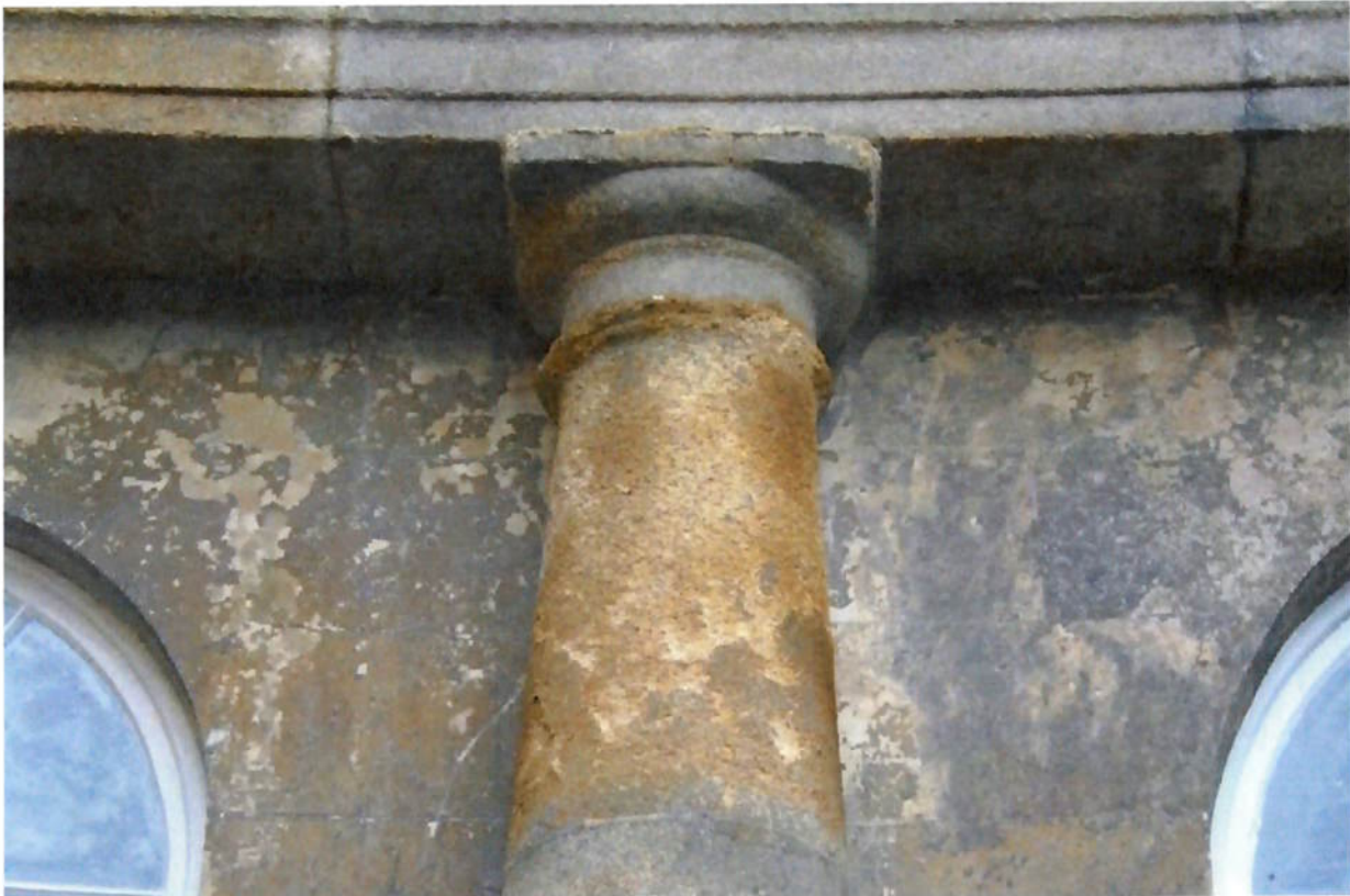
Figure 32. Staining to granite
