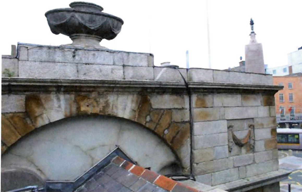
Figure 13. Upper level of the return elevation. Repair to defective lime render required and repointing of joints
