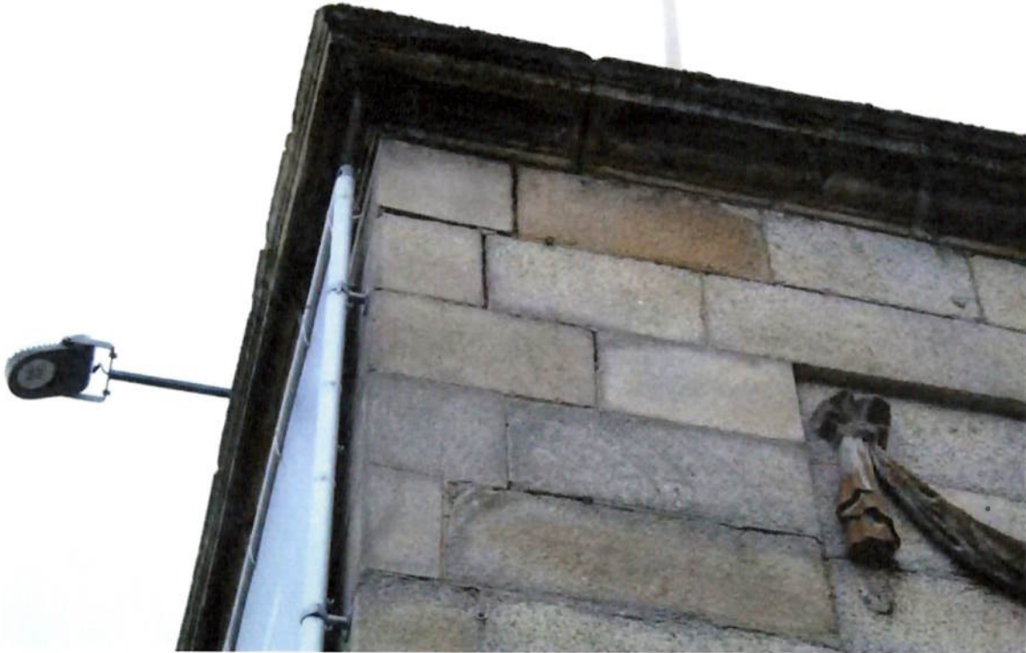
Figure 20 Open joints to the granite stonework to be repointed and missing section of swags to be replaced.
