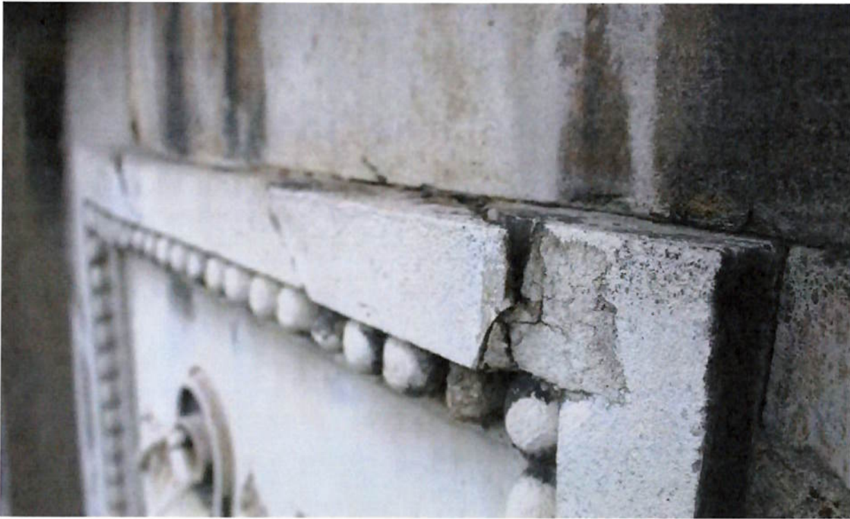
Figure 13. Corrosion of fixings causing stone damage to Portland limestone panels.
