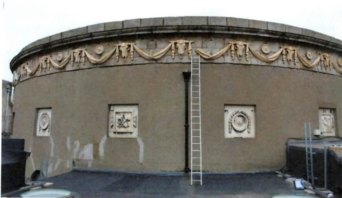
Figure 4. Elevation view of the rotunda theatre building. It is proposed that the missing Coade stone rounder and sections of swags are replaced and the cement render that is cracked and repaired is hacked off and re-rendered.
