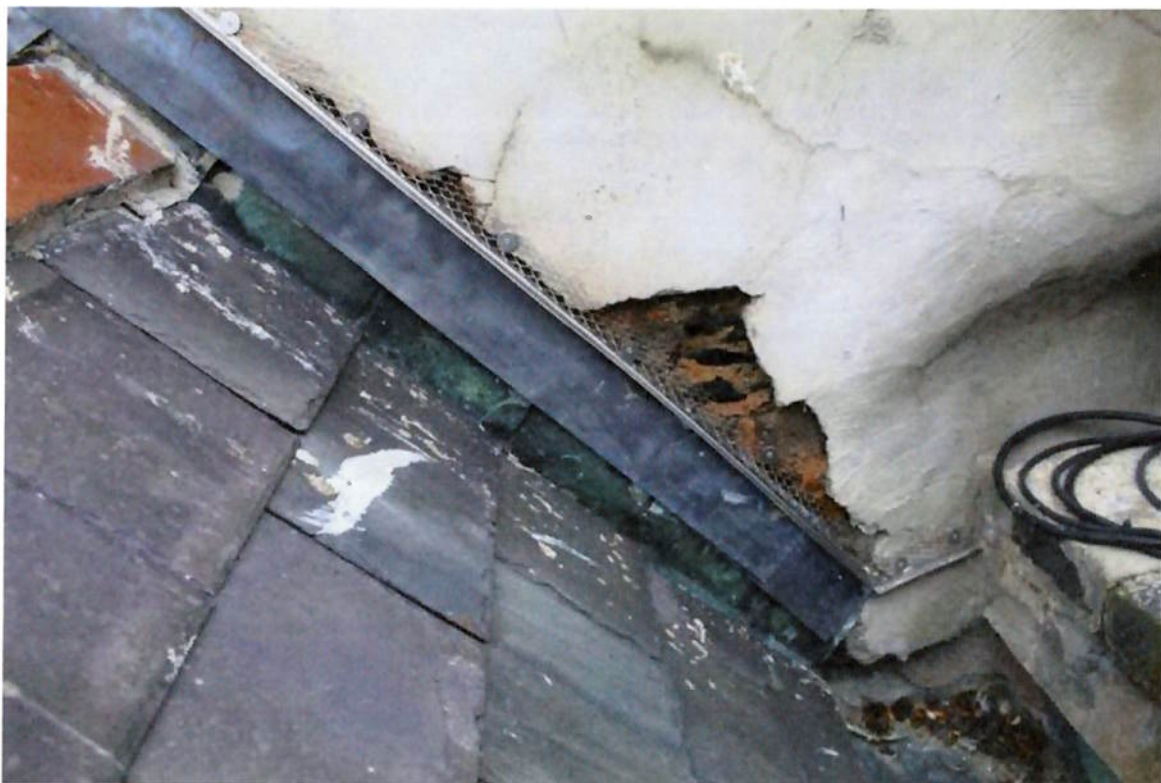
Figure 14. Defective (lime) render and flashing allowing water ingress. To be hacked off and re-done in lime render
