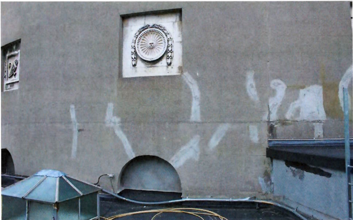
Figure 11. Defective render at roof level.
