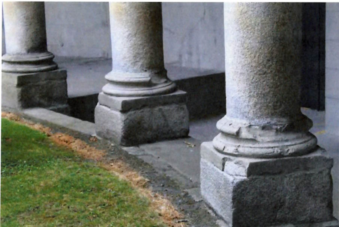
Figure 18. Deteriorating render repairs to column bases. Defective cement-render to be removed and replaced by moulded granite indents to match original.
