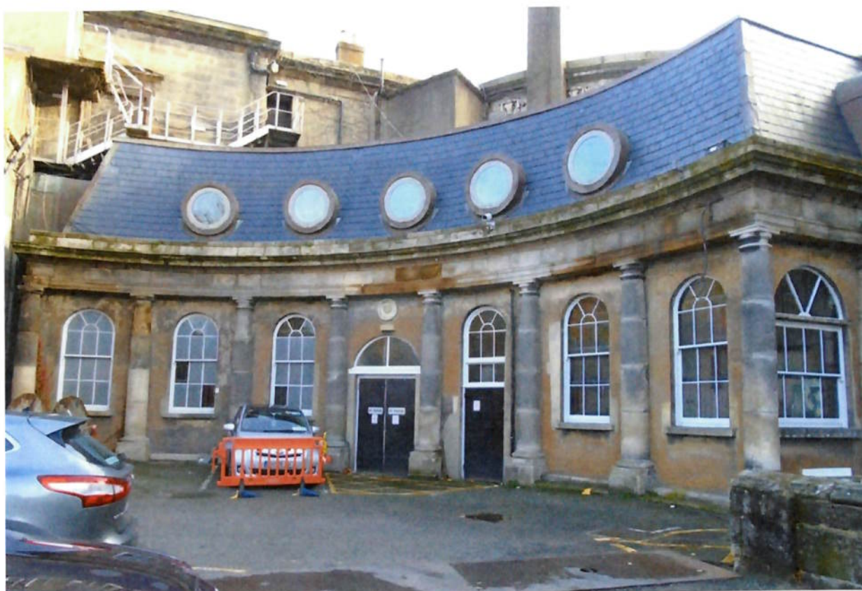
Figure 29. The roof is under separate ownership. Evidence of cleaning trial by Thomann Hannery samples on two columns on left hand side. Like the front elevation, this has proved to be too severe and a gentle steam clean will be used instead
