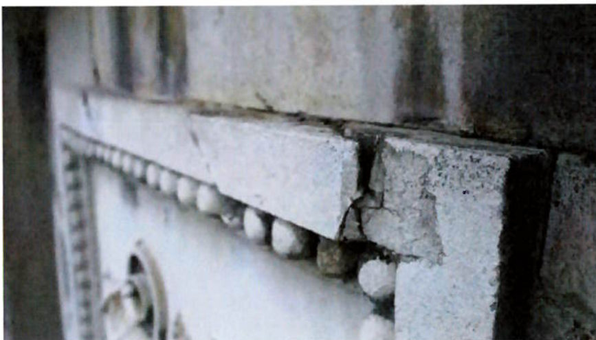
Figure 10. Corrosion of fixings causing stone damage to Portland limestone panels.
