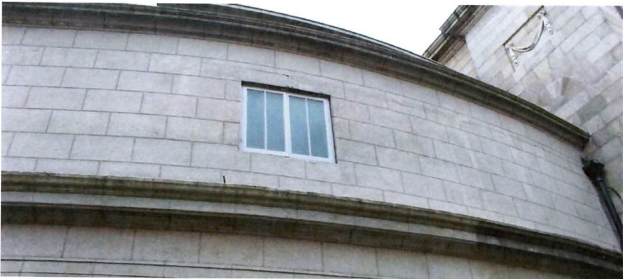
Figure 26. Continuation of the horizontal cracking to the East Elevation.
